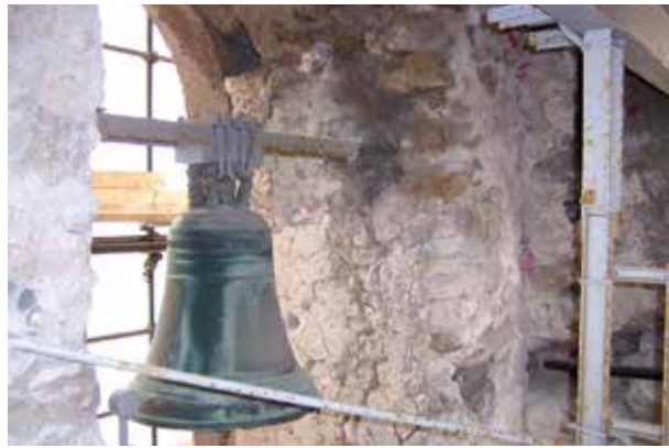
Figs. 57-58 Photo of the internal preservation state of the Bell Tower masonry structure before the 2004 consolidation works when the preservation state of the masonries, the ladder and the bell bearing structure came out.
