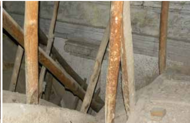
Figs. 23-25 Photos of the wooden structure of the barrel vault overlooking the central nave of the Main Church and the original tuff structure made of a strong entablature and ionic capitals.
